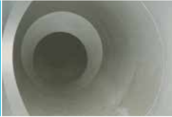
Internal Circle Water Pipe
