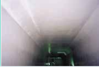
Internal Condensed Cooling Water Conduit
